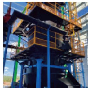
First Industrial scale gasification plant of olive pomace in the olive oil industry. As courtesy of Bioliza
